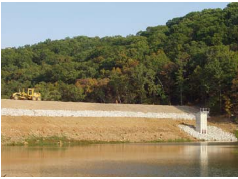
Construction of the dam is shown here nearly complete. The tower on the right is the outflow tower. The new lake level will be to the top of the tower, raising the water level 9 feet from it's original height to be level with the row of white rocks along the length of the dam.
