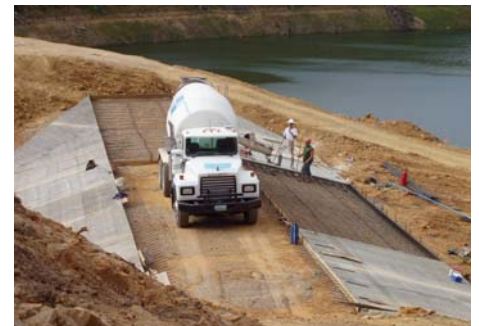
Shown in it's construction faze is the new emergency overflow spillway for our new dam. During heavy rains the excess water will flow quickly over this spillway thereby saving the integrity of the dam.
